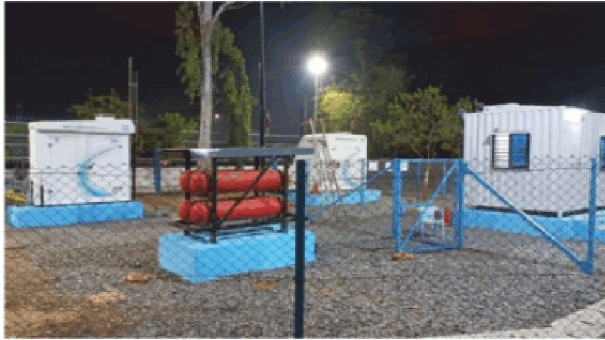
(NTPC Kawas Green H2 Blending project having electrolyser, hydrogen storage and blending skid)
